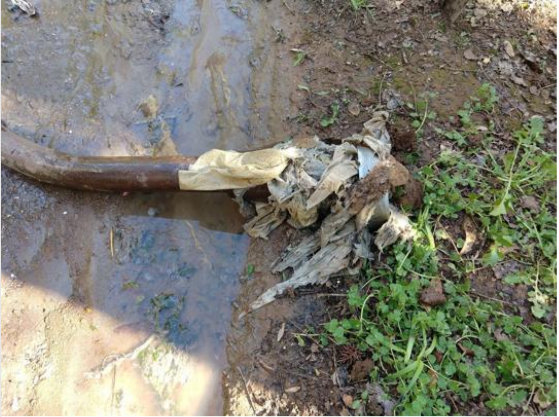
Wet wipes wreak havoc on Athens-Clarke County sewage system
